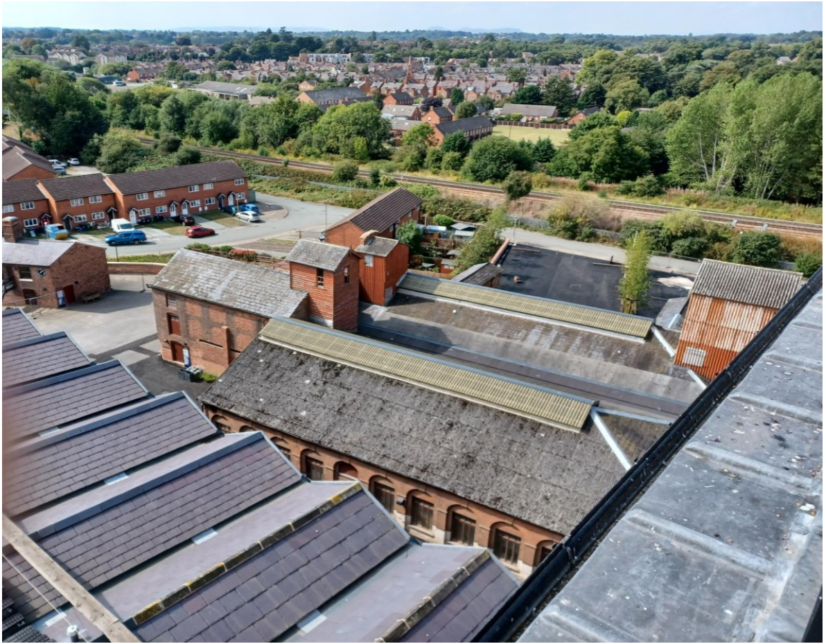
- The view to the South- West off the tower onto the roof of the Flaxmill and Dye House –
